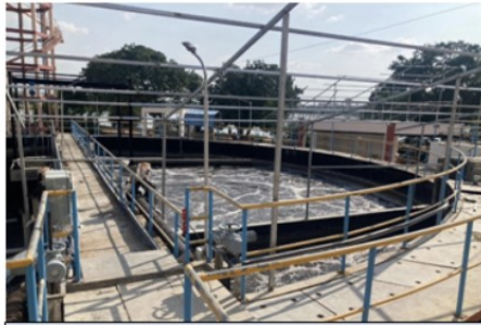
5 MLD Sewage Treatment Plant, Beawar, Rajasthan
